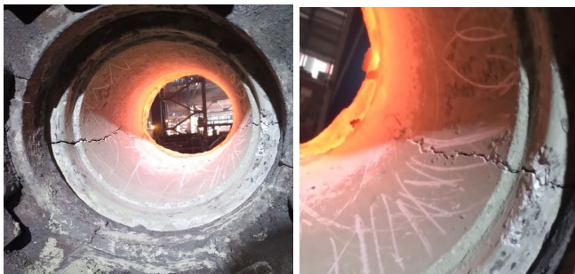
Fig. 11. Cracking observed in seating blocks with regular castable
