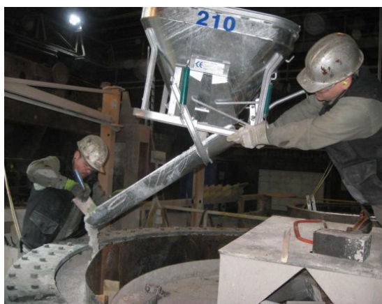
Figure 7: Cast of the lip ring in the steel ladle with Sol-Gel material
